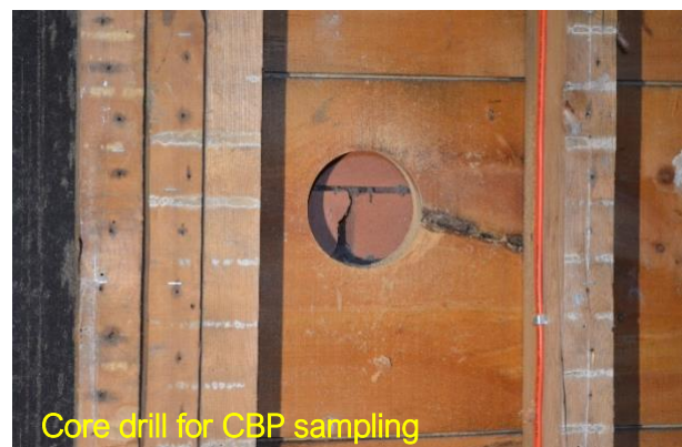
Damaged trusses of addition
